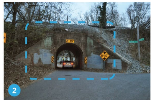
Blount Ave - narrow railroad underpass creates a traffic bottleneck
