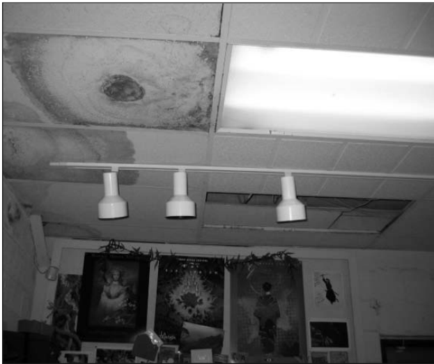
Water damaged ceiling tiles, before...
