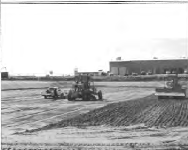
Photograph of the site being compacted with clean fill. Polyvinyl chloride liner can be seen around the edges of the site.
